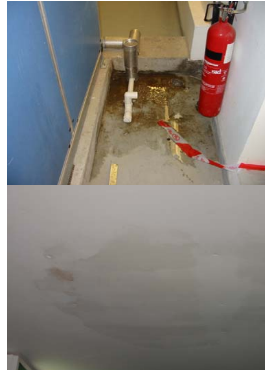
Active water leakage in Air Handling Unit (AHU) room and the wet ceiling below the AHU room
