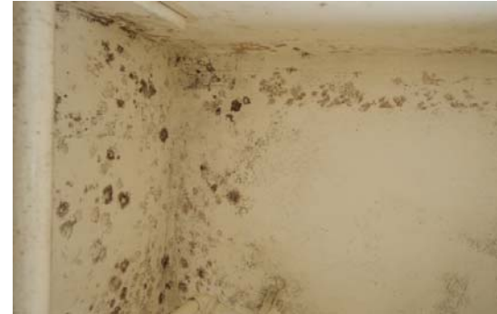
Mould growth on the walls of a non-ventilated stair well
