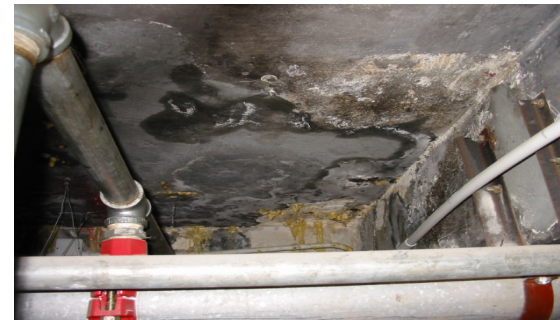
Mould growth on the ceiling due to flooding in the past
