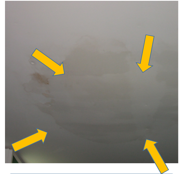
Water stain with a thin layer of mould growth on the ceiling
