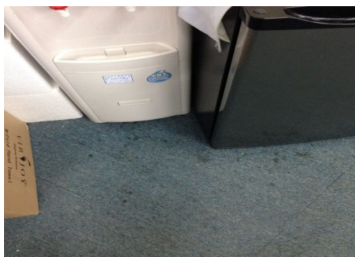
Figure 2.1e: Mould growth on carpet next to water dispenser
