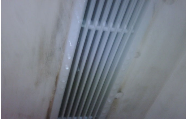
Figure 2.2a: Condensate on air diffuser surface
