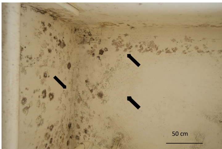
Figure 2.1a: Patches of observable mould (arrows) on a painted cement wall
