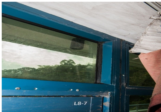
Figure 2.3e: Past water damage on ceiling next to an improperly sealed door
