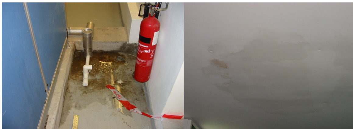
Figure 2.3a: Active water leakage in Air Handling Unit (AHU) room and the wet ceiling below the AHU room
